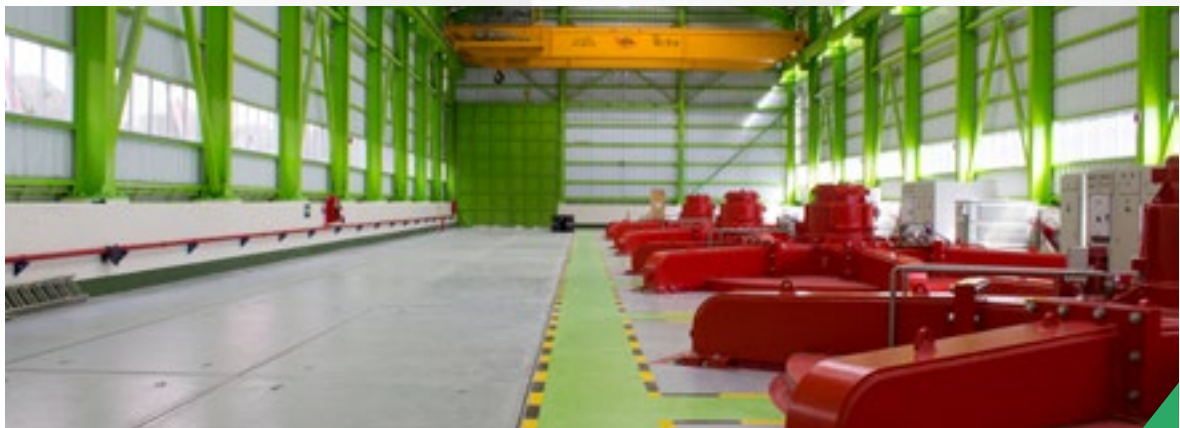
1,100 MW in Pelton, Kaplan and Francis Turbines
